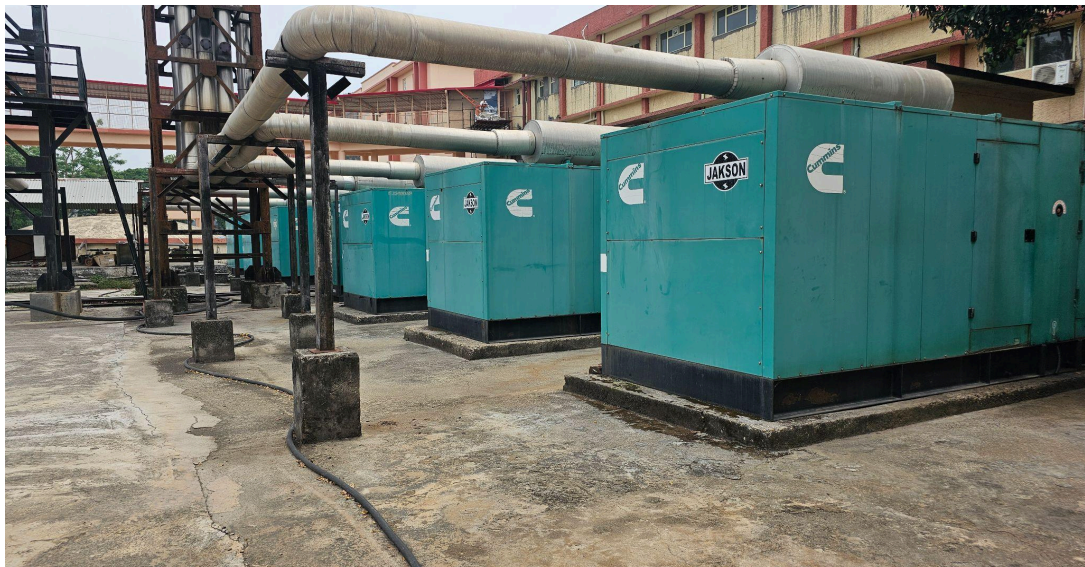
9 Diesel generator sets with Automatic Mains Failure panels and load synchronization system
