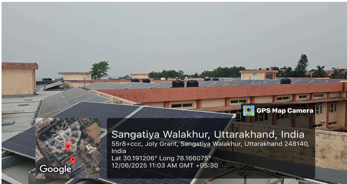
Rooftop solar panels at Swami Rama Himalayan University harnessing renewable energy to promote sustainability and reduce carbon footprint.
