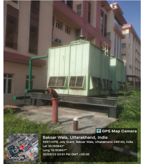
BEE star rated energy efficient AC package unit supporting HVAC system
