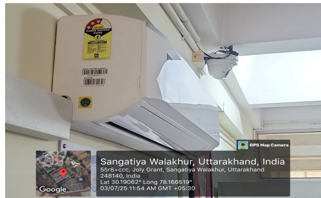
Energy Efficient split inverter air conditioner
