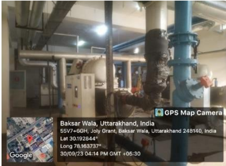
HVAC system installed in the University
