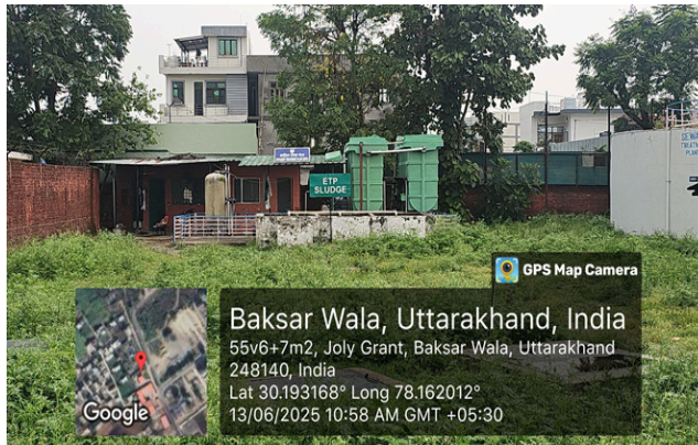
Effluent Treatment Plant (Capacity 90,000 liters per day)
